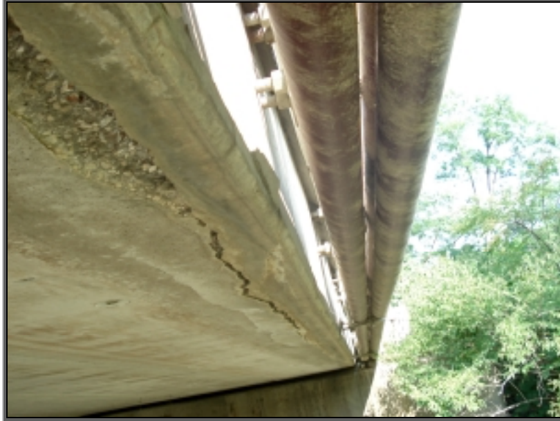
River Ridge Lane Bridge #00.170 - underside view, severe cracking
