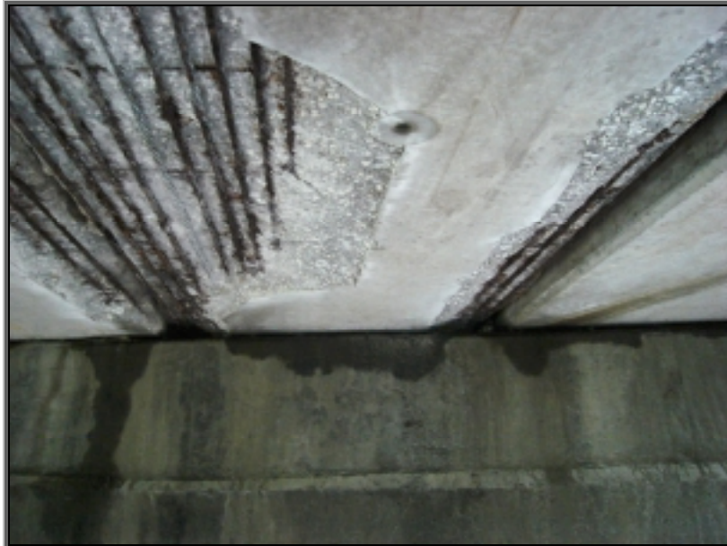
River Ridge Lane Bridge #00.170 - underside view, exposed rebar
